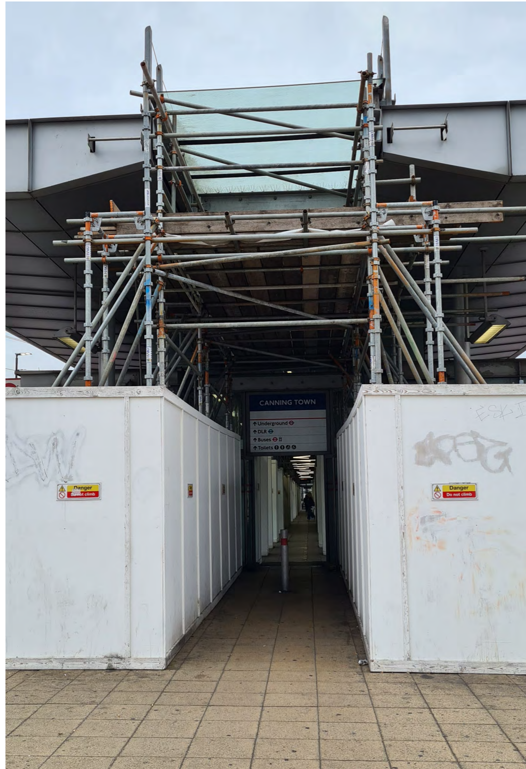
Figure 2: External view of Canning Town Bus Station entrance showing scaffolding in place under the glazed canopy.
