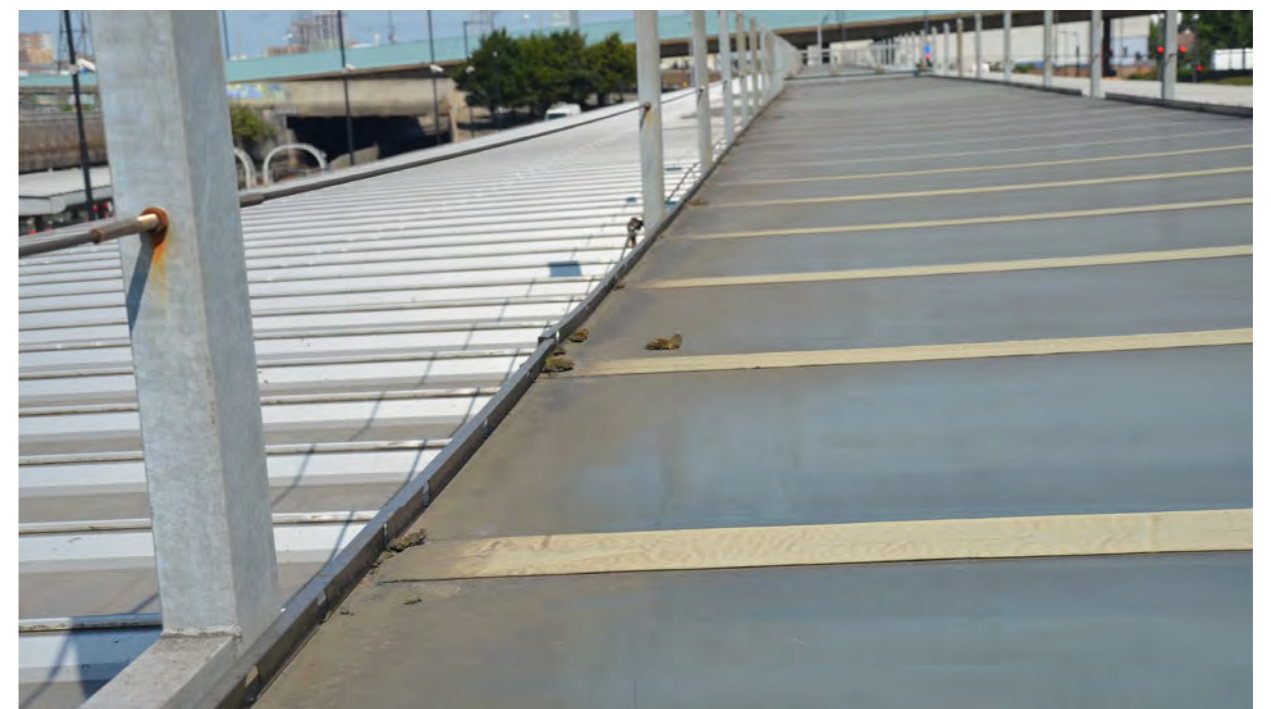
Figure 8: Glazed roof canopy with access restrictors to prevent persons stepping on the glass panels.
