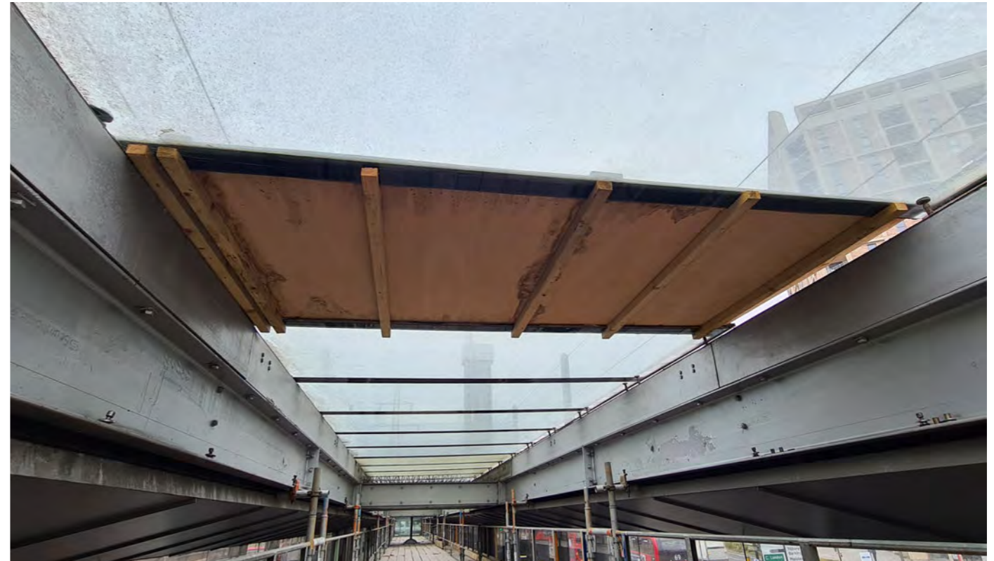
Figure 3: The broken glass panel has been replaced with plywood board.
