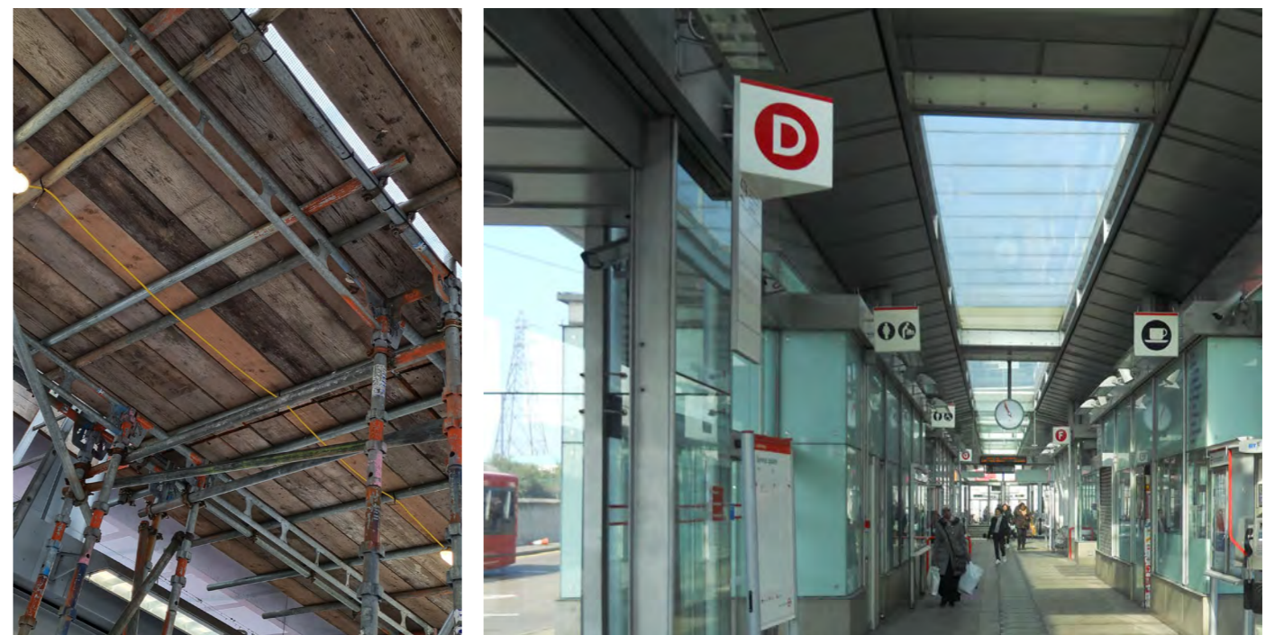
Figures 4-5: Left: Scaffolding structure viewed from inside the station. Right: Station interior prior to breakage.
